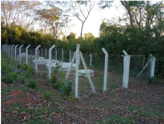
Figure 13: Machado Campus sewage treatment system with septic tank, anaerobic filter and sink.
