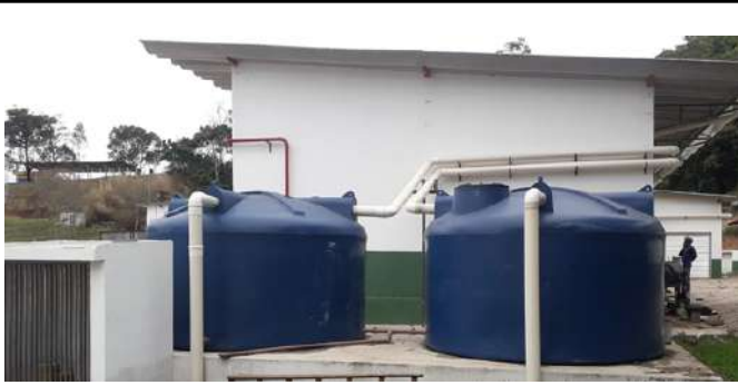
Figure 13: Carmo de Minas Campus rainwater reservoir tanks.
