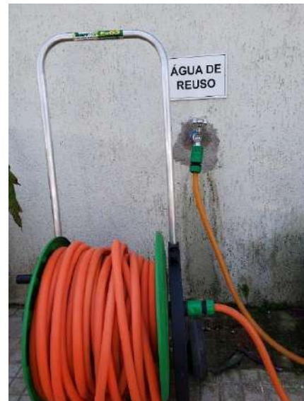
Figure 18: Rectory sign indicating reused water tap.
