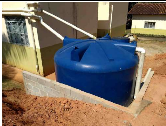
Figure 5: Inconfidentes Campus rainwater reservoir tank.
