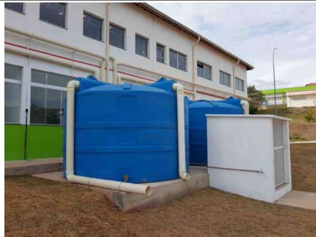
Figure 10: Pouso Alegre Campus rainwater reservoir tanks.
