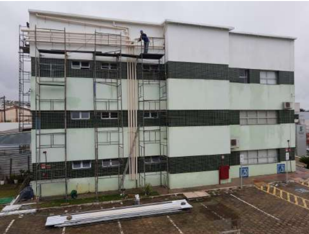
Figure 19: Rectory new rain harvesting system.
