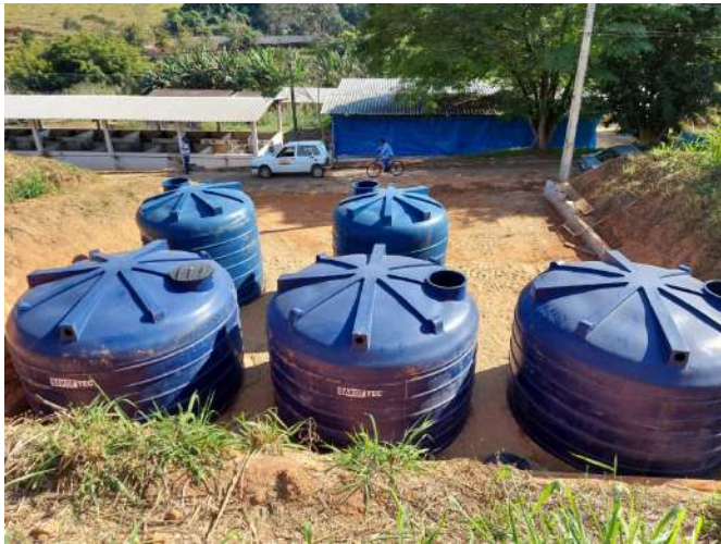
Figure 17: Machado Campus new rainwater reservoir tanks.
