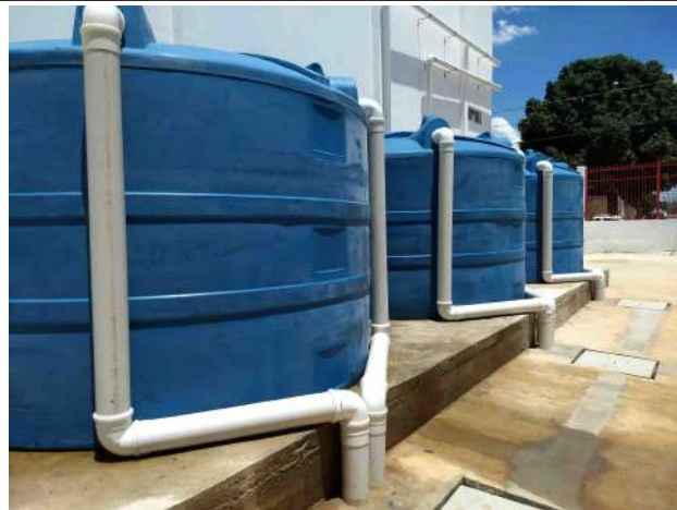
Figure 8: Passos Campus rainwater reservoir tanks.
