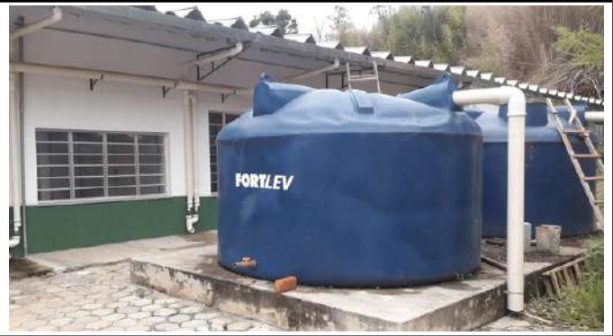
Figure 14: Carmo de Minas Campus rain harvesting system.
