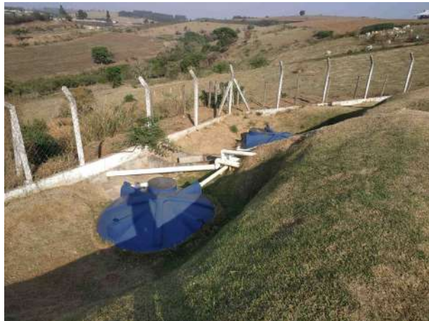
Figure 7: Muzambinho Campus rainwater reservoir tanks.
