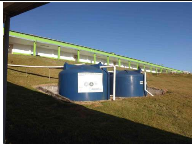
Figure 6: Machado Campus rainwater reservoir tanks.
