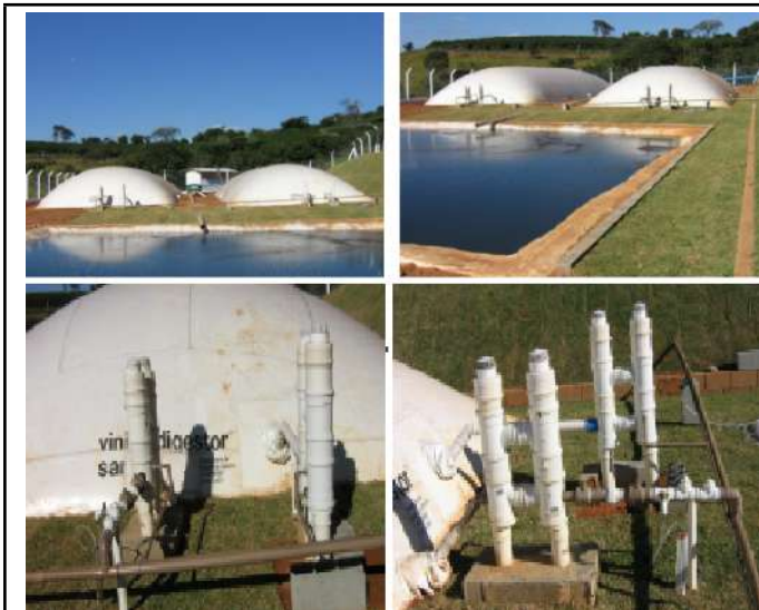
Figure 1: Muzambinho Campus swine waste treatment.
