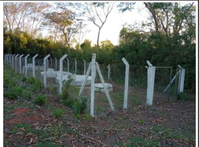
Figure 12: Machado Campus sewage treatment system with septic tank, anaerobic filter and sink.
