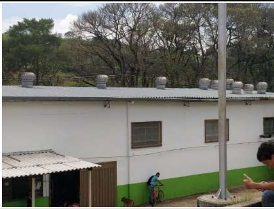
Figure 15: Campus Machado Coffee Roasting Building exhausters.
