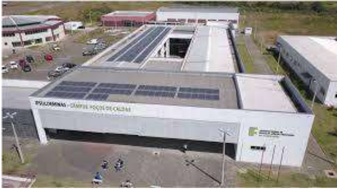
Figure 5: Campus Poços de Caldas solar power plant.
