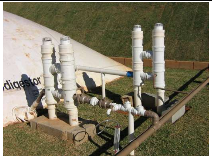
Figure 14. Swine waste treatment unit for biogas production.
