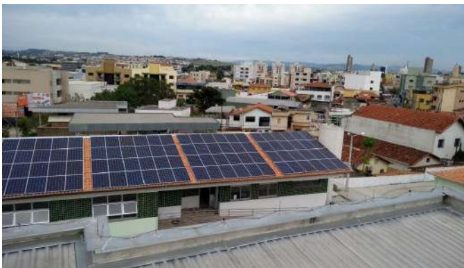
Figure 9: Rectory solar power plant.
