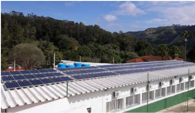
Figure 7: Campus Carmo de Minas solar power plant.
