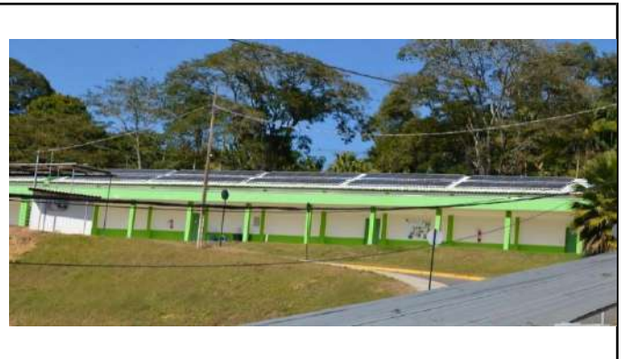
Figure 2: Campus Machado solar power plant.
