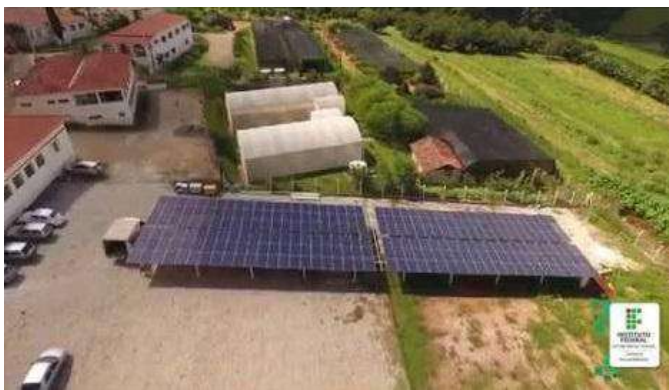
Figure 3: Campus Muzambinho solar power plant.
