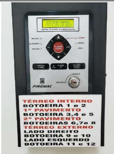
Figure 3: Rectory fire-fighting system – Fire alarm.
