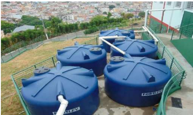
Figure 7: Campus Três Corações rainwater recovery system for covering the flushing and irrigation – Water storage tanks.
