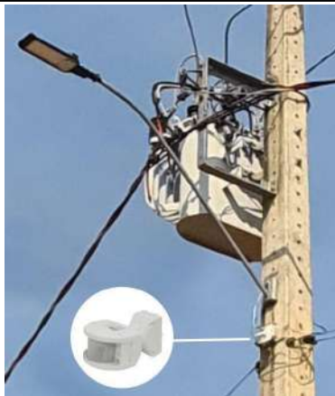
Figure 19: Machado Campus motion detectors installed on street lights.
