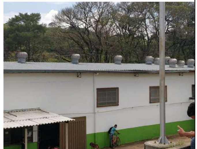
Figure 10: Campus Machado passive cooling and/or exploitation/limitation systems for free supplies – Coffee roasting building exhausters.
