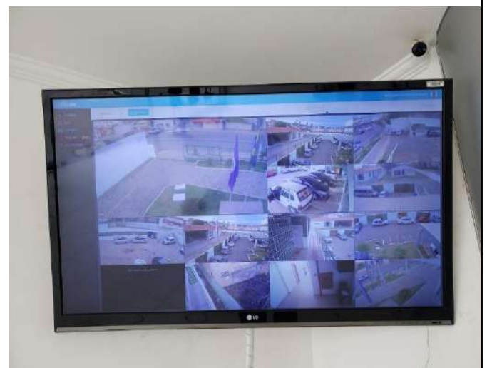
Figure 4: Rectory video surveillance system – Camera control.
