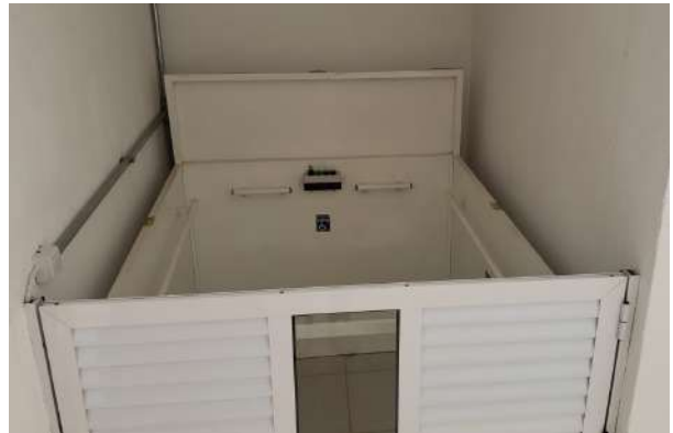
Figure 14: Poços de Caldas Campus elevator for people with special needs.
