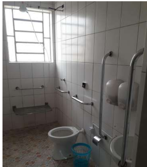
Figure 16: Inconfidentes Campus accessible toilet and shower for people with special needs.
