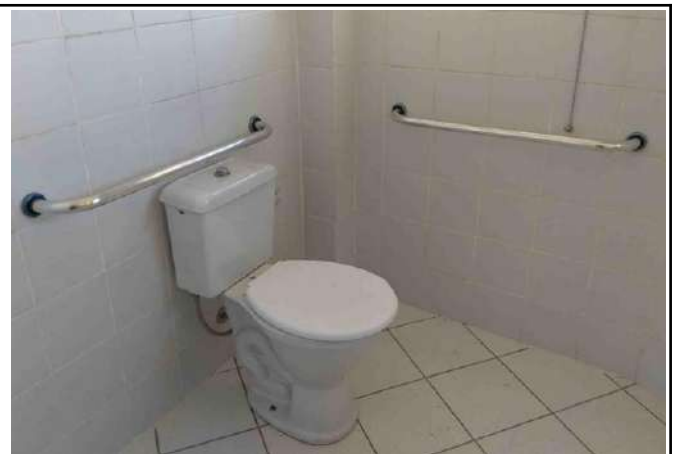
Figure 2: Rectory toilet water box flush.
