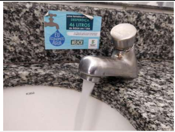
Figure 6: Campus Machado tap with faucet aerator.
