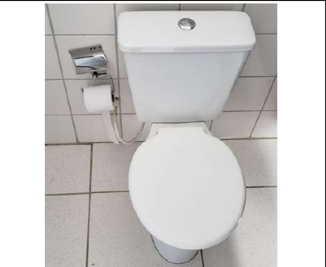
Figure 14: Poços de Caldas Campus toilet flushing with double activation.
