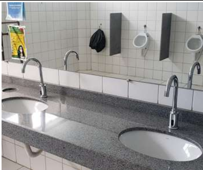
Figure 13: Poços de Caldas Campus auto-sensor activated water taps.
