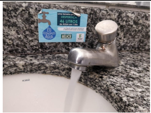
Figure 6: Campus Machado tap with faucet aerator.
