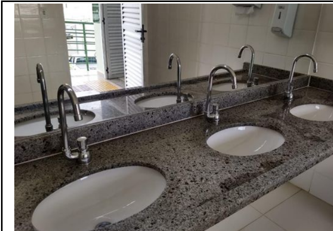
Figure 1: Rectory time delay water taps.
