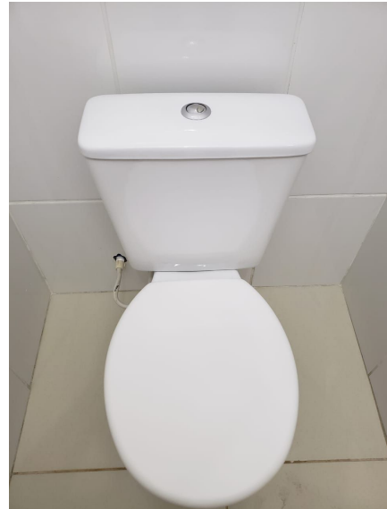
Figure 10: Rectory toilet water box flush with double drive.
