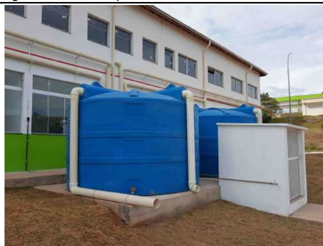
Figure 10: Pouso Alegre Campus rainwater reservoir tank.
