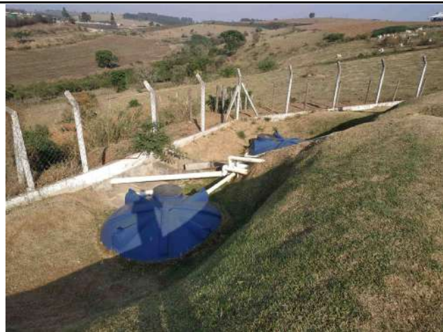
Figure 7: Muzambinho Campus rainwater reservoir tanks.
