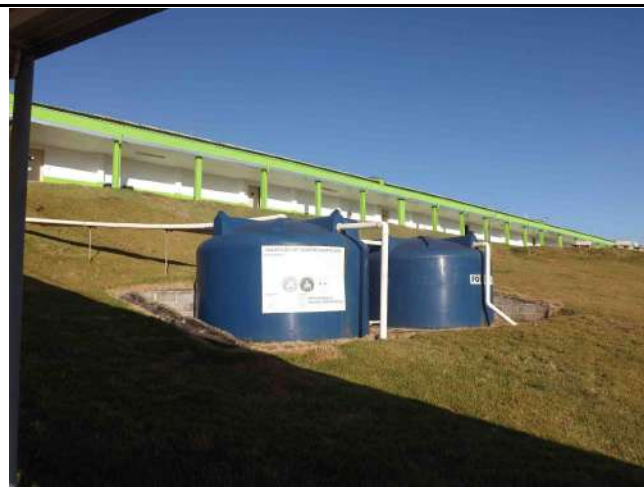
Figure 6: Machado Campus rainwater reservoir tanks.
