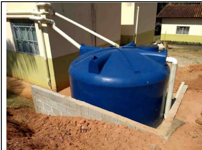
Figure 5: Inconfidentes Campus rainwater reservoir tank.
