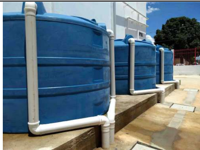
Figure 8: Passos Campus rainwater reservoir tanks.
