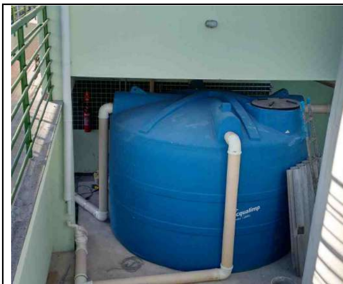
Figure 13: Rectory rainwater reservoir tank.
