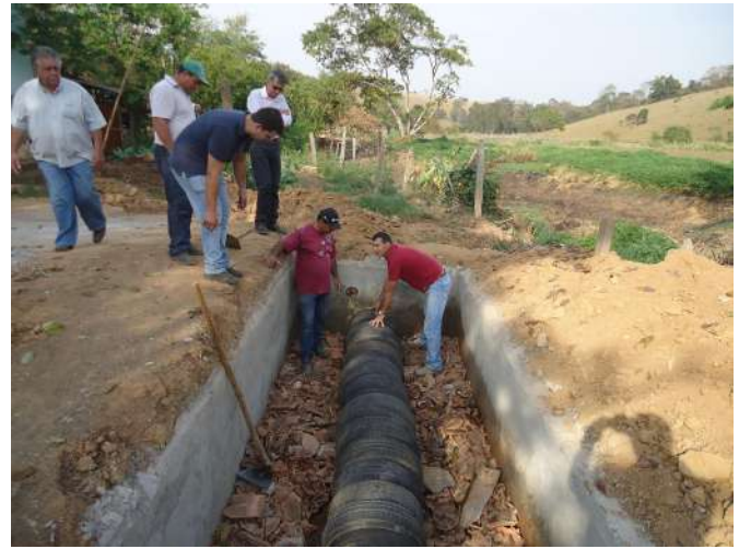
Figure 8: Inconfidentes Campus Milk Cattle sector ecological septic tank.
