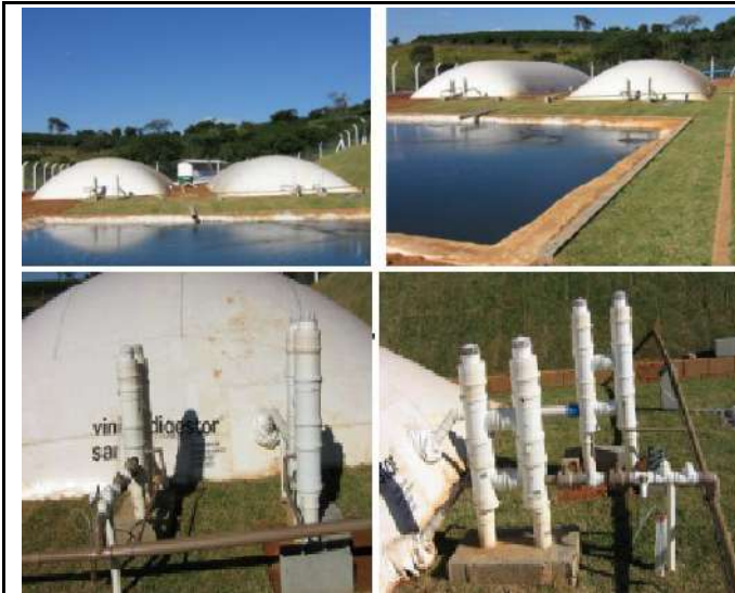
Figure 1: Muzambinho Campus swine waste treatment.
