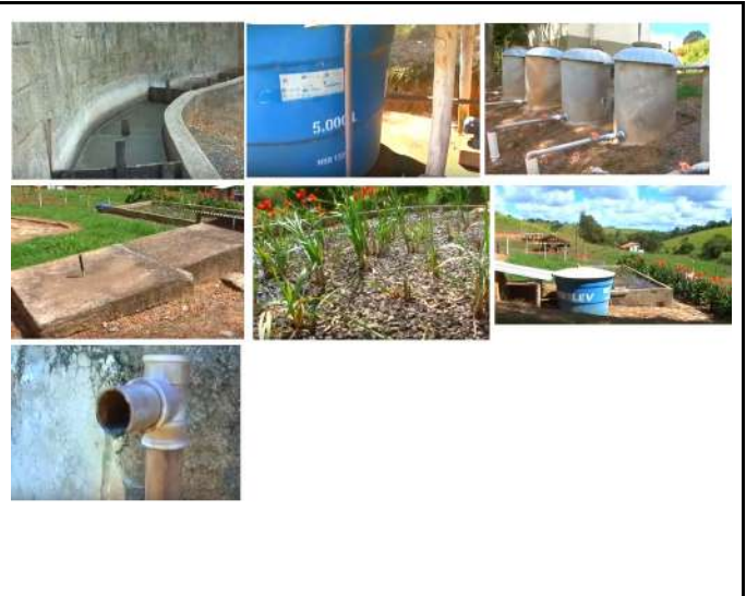
Figure 2: Inconfidentes Campus livestock waste treatment.
