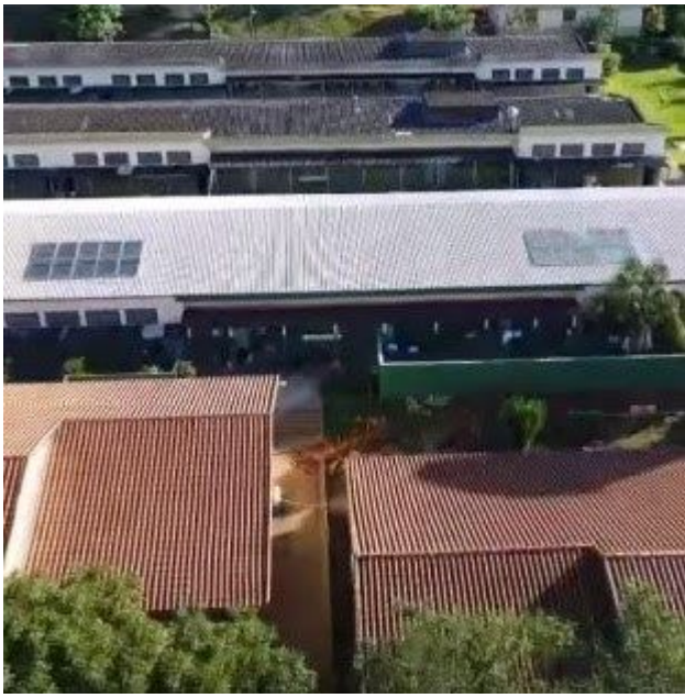
Figure 15. Inconfidentes Campus Solar water heating system.
