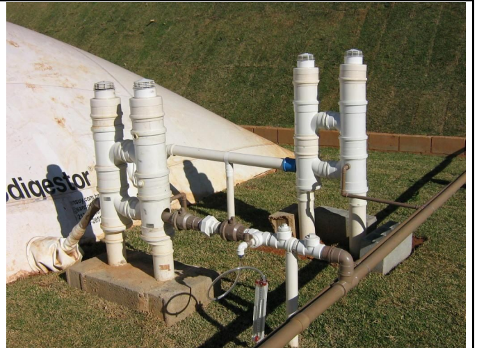
Figure 14. Swine waste treatment unit for biogas production.
