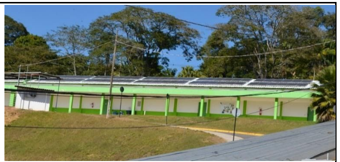
Figure 2: Campus Machado solar power plant.
