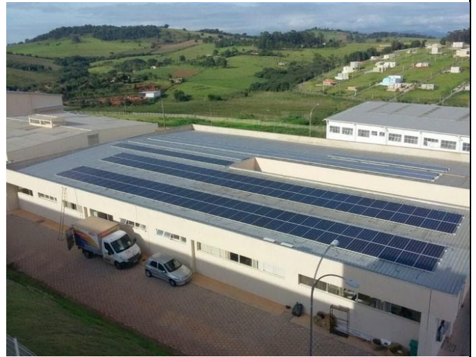
Figure 6: Campus Pouso Alegre solar power plant.
