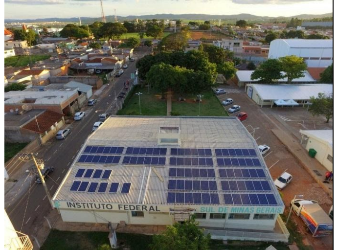
Figure 4: Campus Passos solar power plant.
