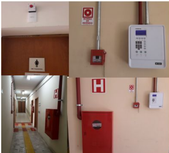
Figure 21: Inconfidentes Campus motion detector and fire-fighting system.
