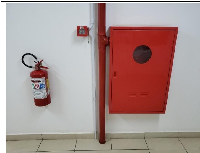
Figure 1: Rectory fire-fighting system – Fire extinguisher and fire hose.
