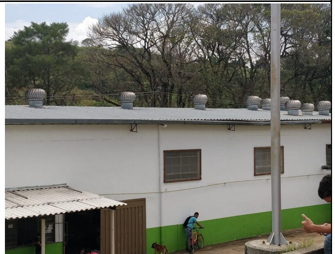
Figure 10: Campus Machado passive cooling and/or exploitation/limitation systems for free supplies – Coffee roasting building exhausters.
