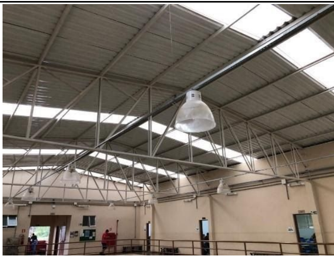
Figure 17: Campus Pouso Alegre passive systems for natural light exploitation – Engineering building.
