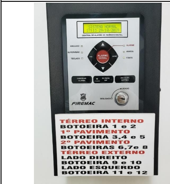
Figure 3: Rectory fire-fighting system – Fire alarm.
