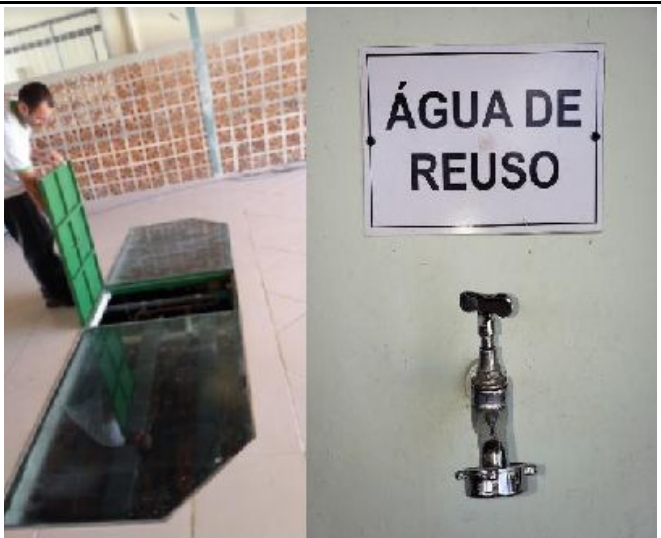
Figure 9: Rectory rainwater recovery system for covering the flushing and irrigation – Water storage tank and reuse water tap.
