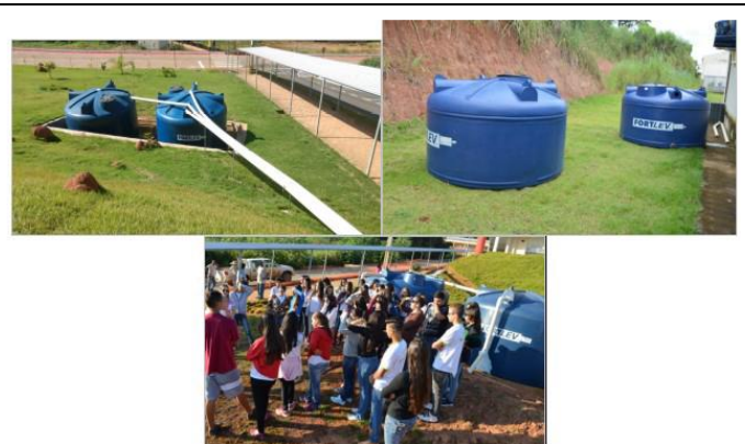
Figura 2 Campus Machado - Rain Harvesting System
