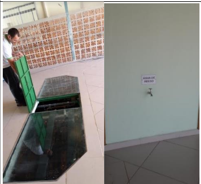
Figura 4 Water Management - Rainwater harvesting system and external water tap for reuse
