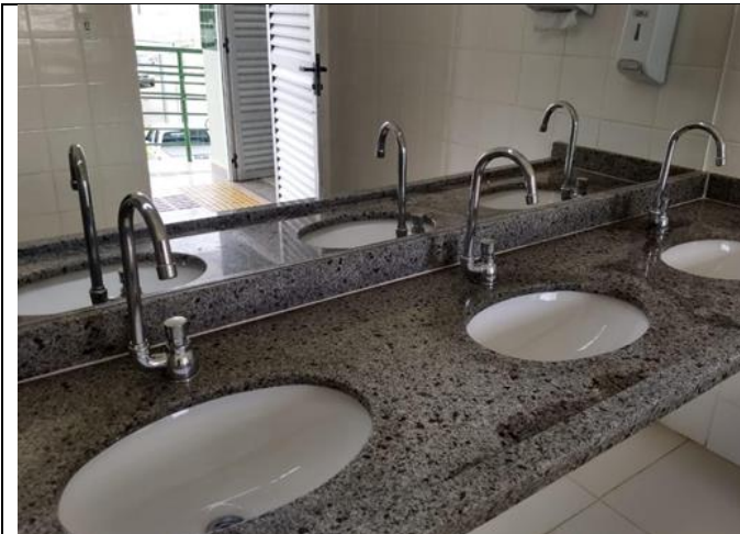
Figure 1: Rectory time delay water taps.
