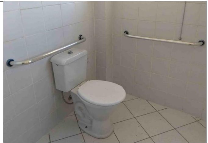
Figure 2: Rectory toilet water box flush.
