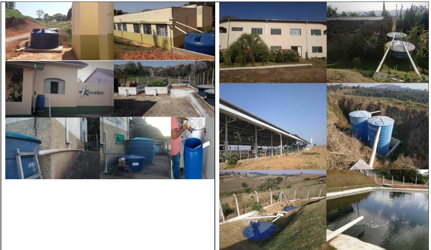
Figure 1: Campus Inconfidentes rain harvesting system.
