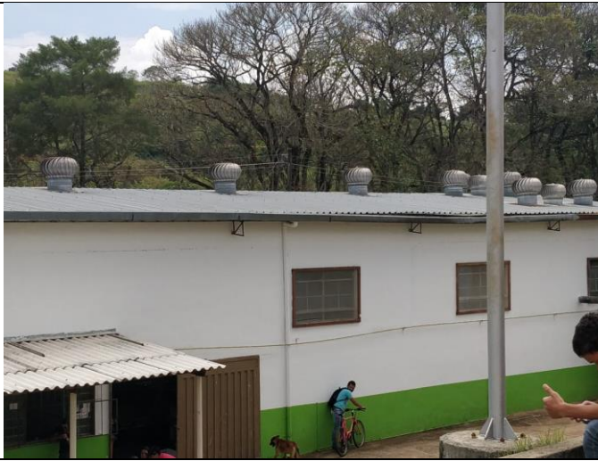
Figure 15: Campus Machado Coffee Roasting Building exhausters.
