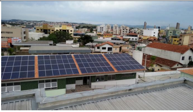
Figure 9: Rectory solar power plant.
