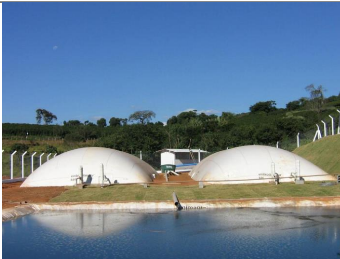
Figure 13. Swine waste treatment unit for biogas production.
