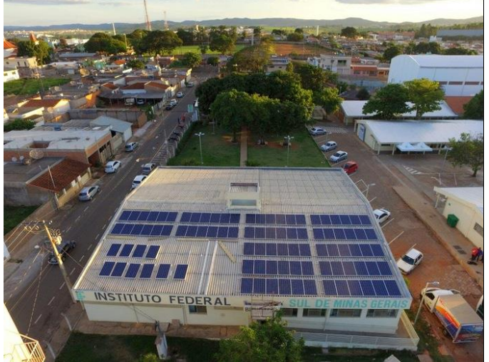
Figure 4: Campus Passos solar power plant.
