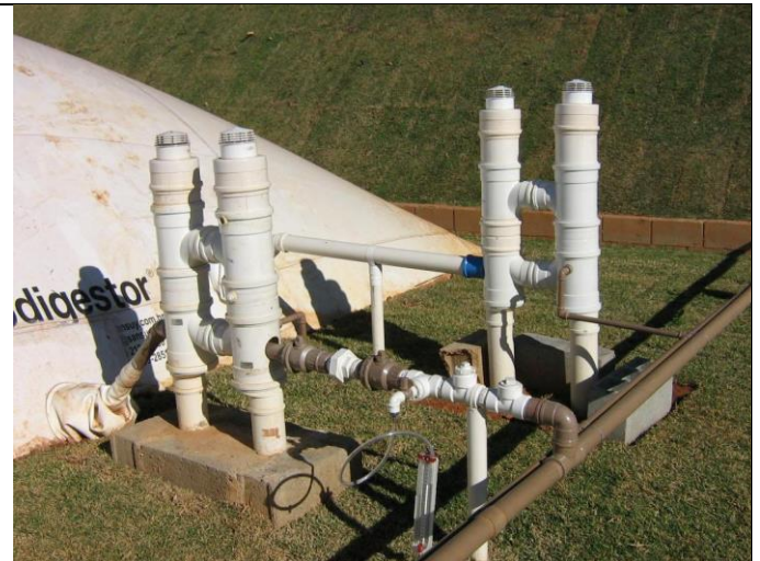
Figure 14. Swine waste treatment unit for biogas production.
