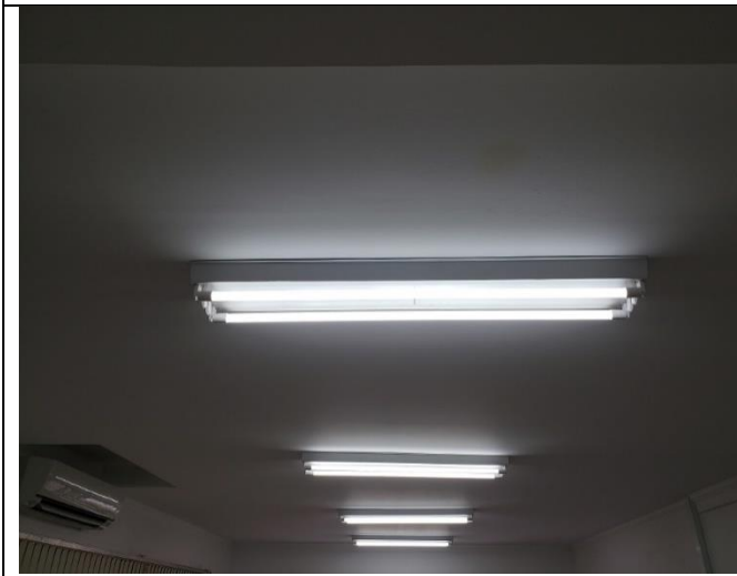
Figure 3: Rectory LED tubular lights.
