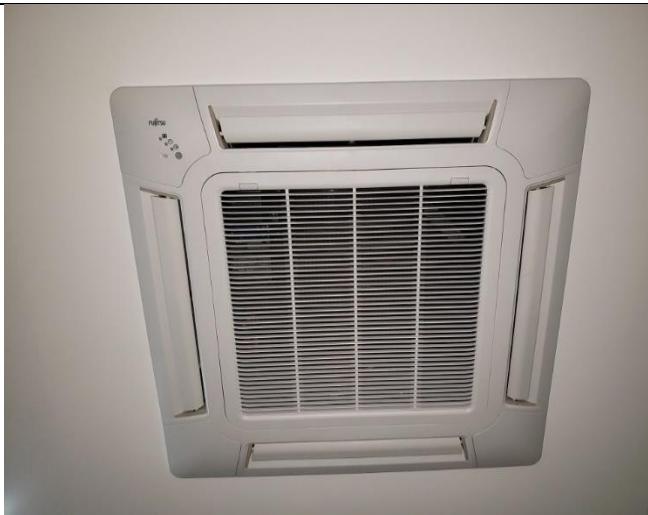
Figure 7: Rectory efficient air conditioning.
