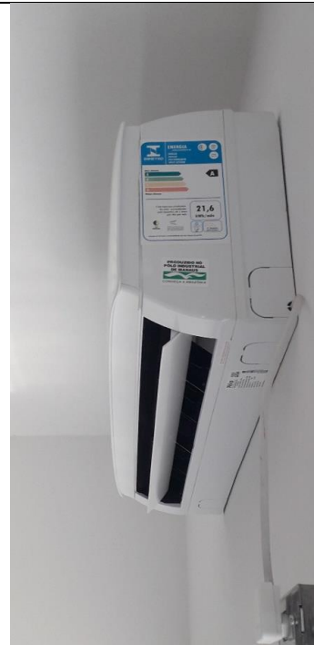
Figure 6: Campus Carmo de Minas efficient air conditioning.
